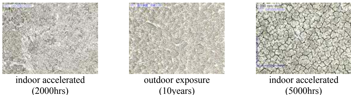
Figure 11. Exposed surface of TPO liner
